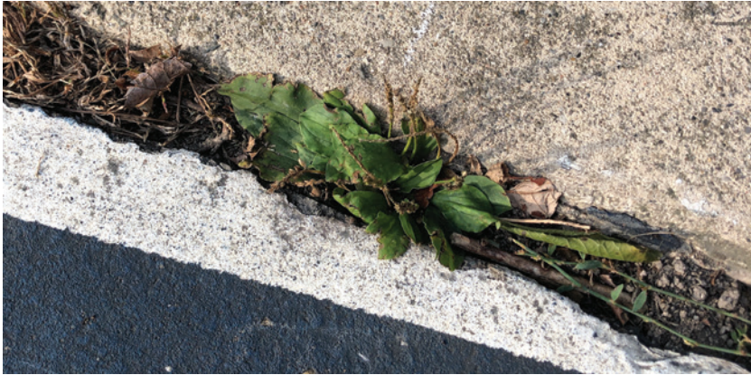
Figure 5.8: Vegblatt ( Plantago ) growing in a crack in a neighborhood basketball court in Ann Arbor, Michigan.
